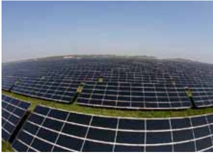
Left and below: Solarpark Waldpolenz (Germany)
