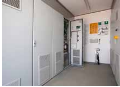
Left: Central inverter
